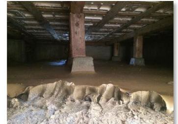
Mud has accumulated under the floor.
