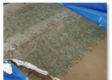
Mold growing behind drywall or engineered wood walls
