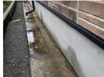
Water is seeping out even though it is not raining.
