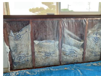
Wet insulation behind walls
